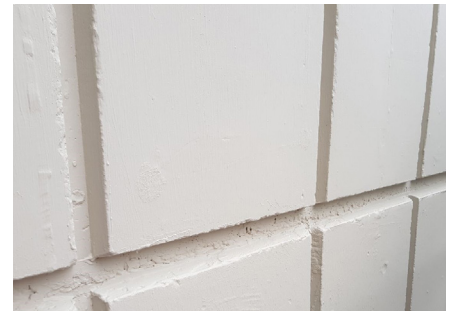
Finished facade with installation of galvanic anodes and anti-carbonation coating to maintain aesthetic appearance.
