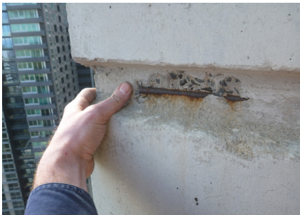
The concrete cover to reinforcement had been significantly reduced due to the presence of architectural false joints.
