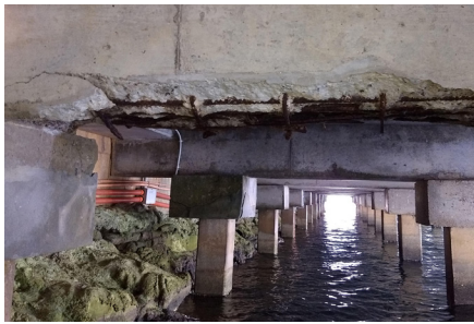
Under the wharf, extensive concrete deterioration and exposed reinforcement.
